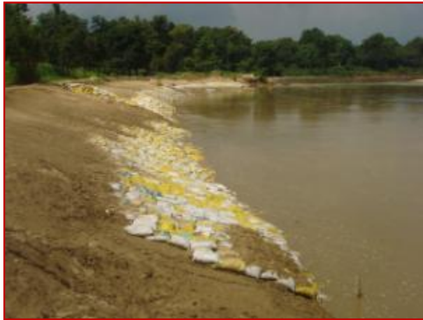
Photo 6: Sand bags on the slope
